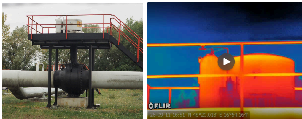
Fig.1: Valve (venting-by-design) - Regulation station 1 Vysoká pri Morave [video link]
